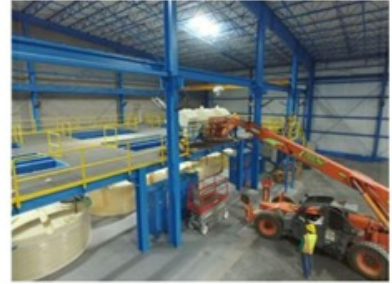
Installed in the AquaRefining Hall
