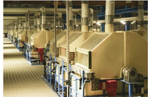
Aqua Metals' AquaRefining Modules at its TRIC facility
